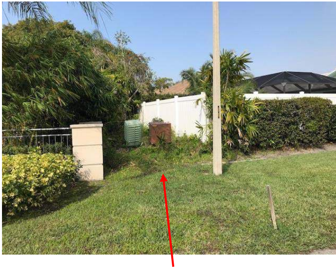
New Plants to be installed
