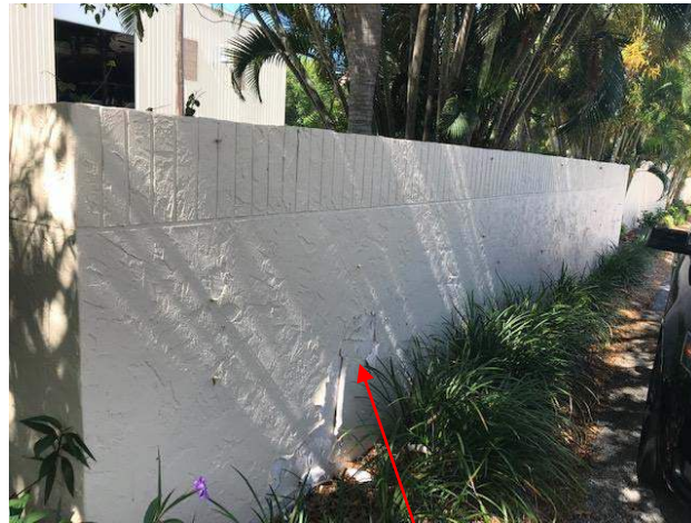
Damage from water – peeling and flaking
